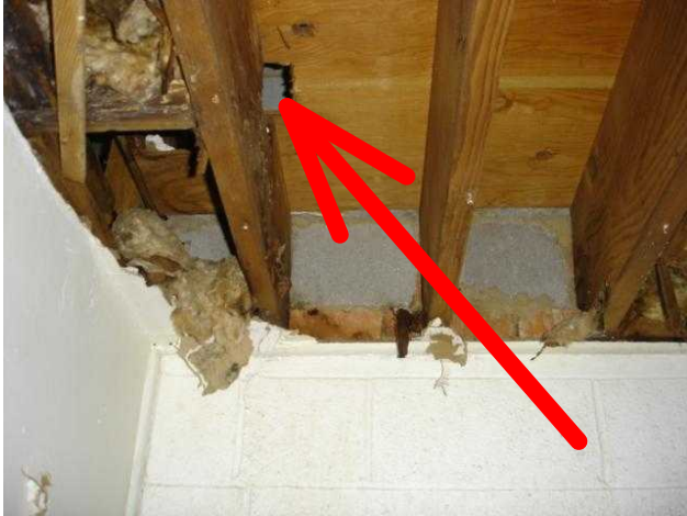
Cut Floor Joist
