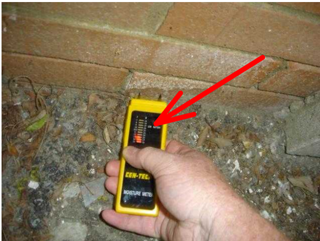
Light shows moisture in the walls on the high side of the meter.
