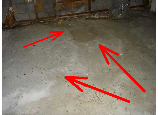
Stress Cracks in the slab with moisture
