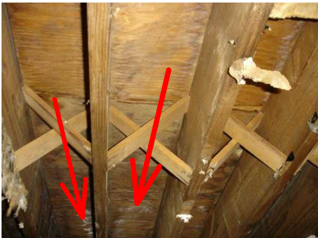
Mold and wood rot
