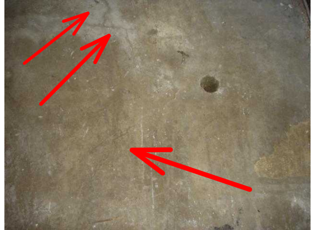
Foundation Slab cracks
