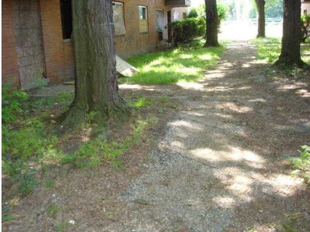
Trees are up-rooting pavement.
