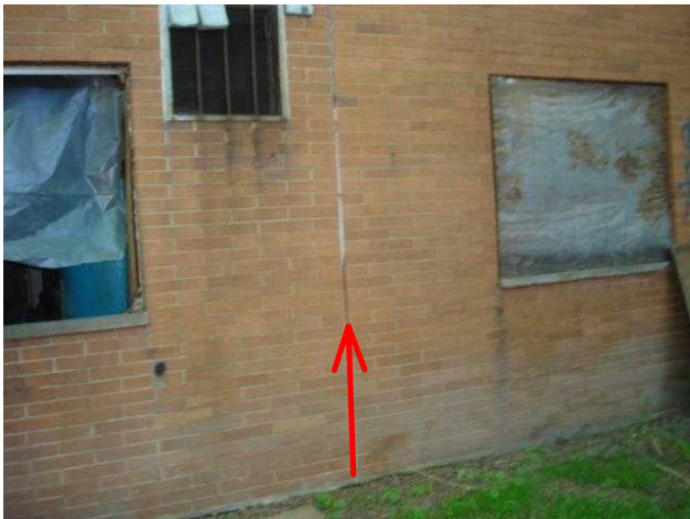
Joints show settlement
