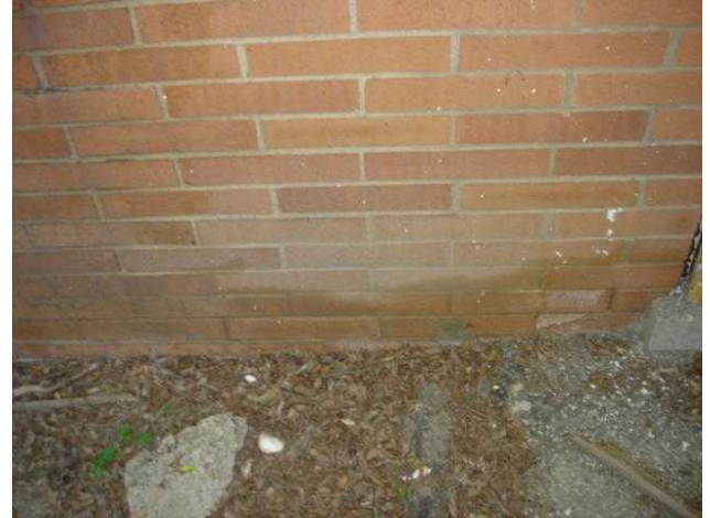
Moisture in the walls
