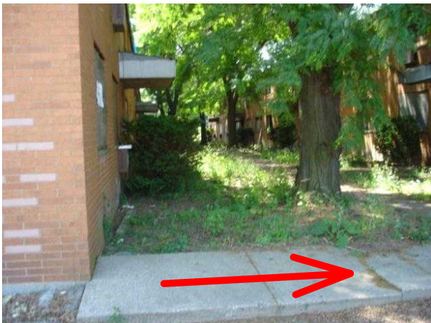
Broken side walks
