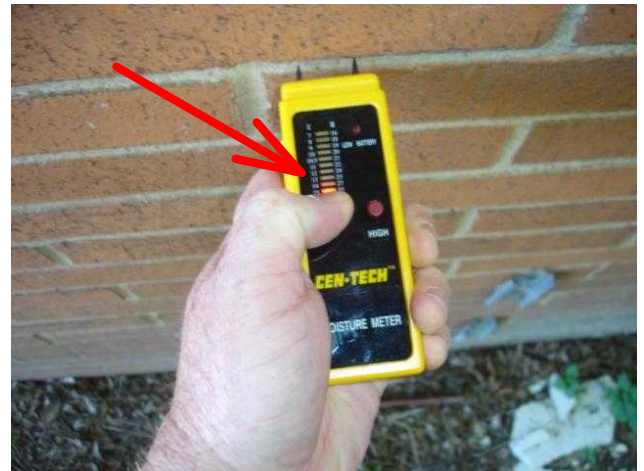
Moisture in the walls
