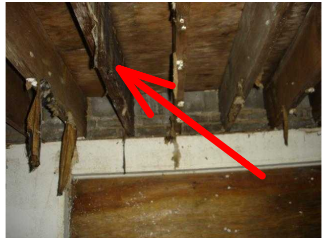
Wood rot in the floor joist
